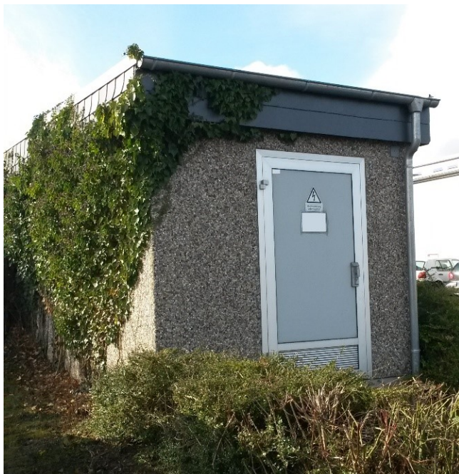
Fig. 11: Measurement site: Transformer station in an industrial estate.
