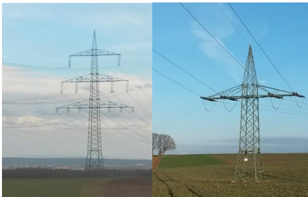
Fig. 4: Measurement sites: 380 kV and 110 kV power lines
